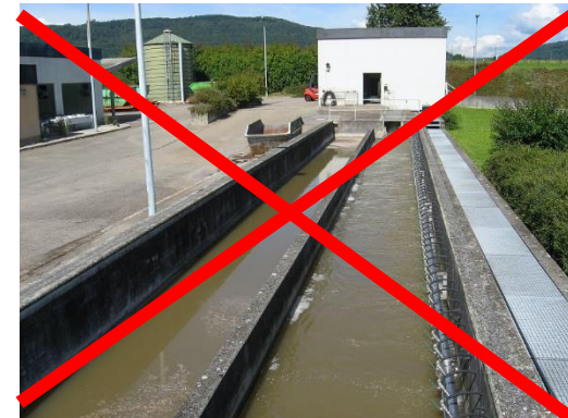
Into the grit trap (not aerated)
