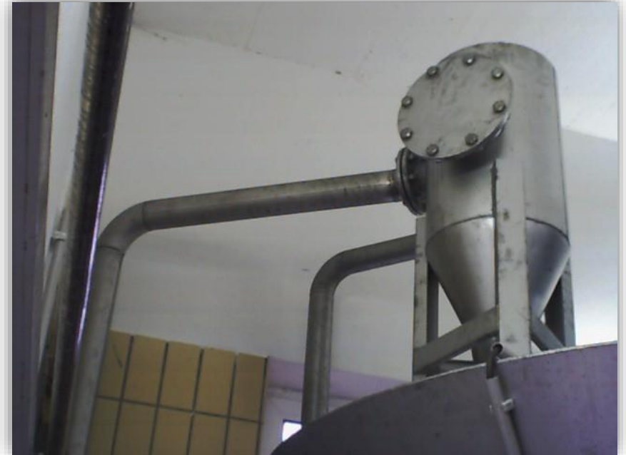
Collection tank with feeding from several lines
