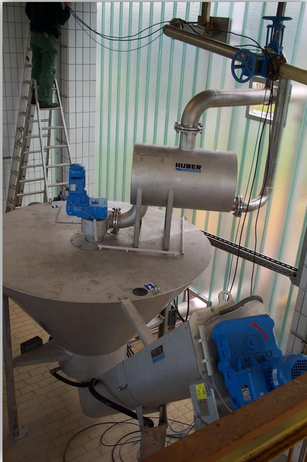
Degasing Tank after an airlift pump
