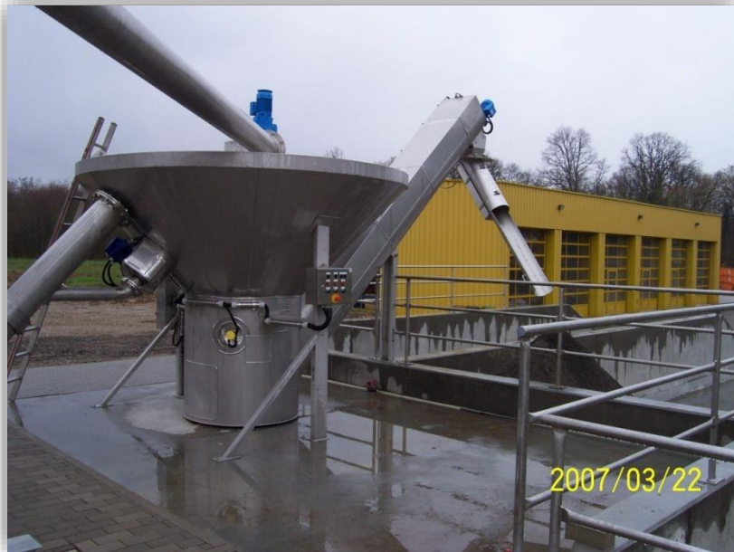
Feeding by a pump system
