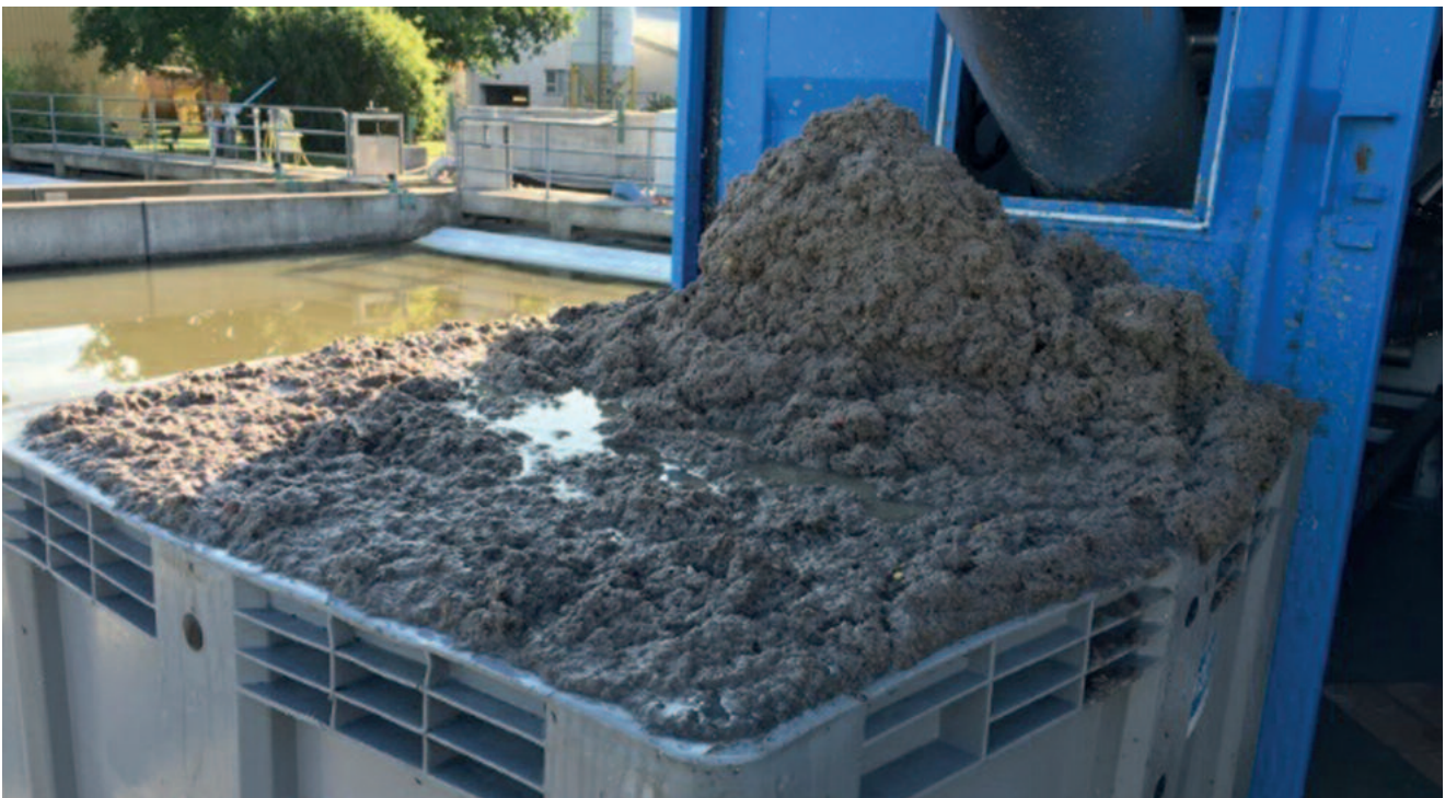
Screenings separated by the HUBER Drum Screen LIQUID mesh: The load to be handled in the biological treatment stage is reduced and more gas can be produced in the digester.
