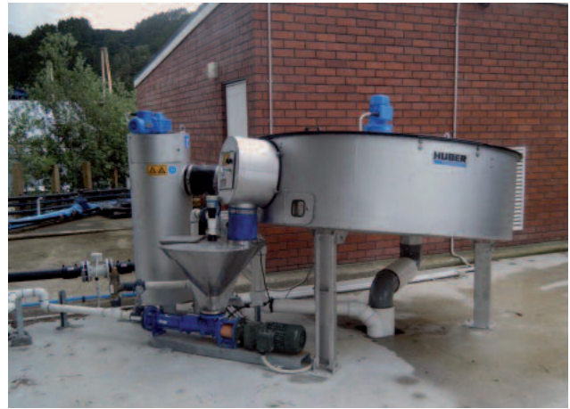
Outdoor installation of a ROTAMAT® Disc Thickener RoS 2S
